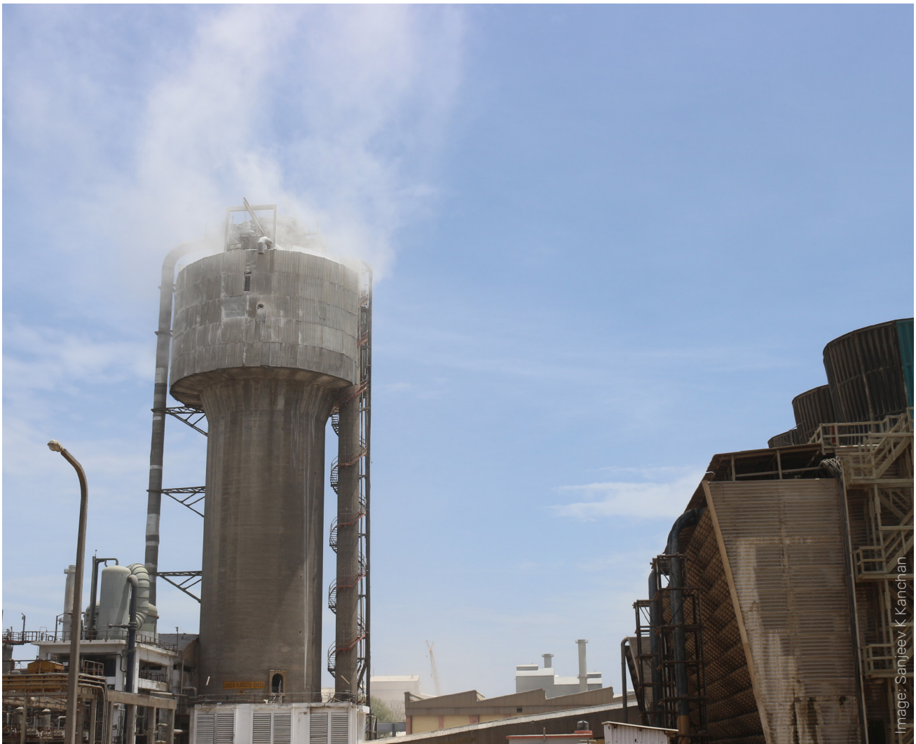
Air emissions from a prilling tower of a Urea fertilizer plant in India.
