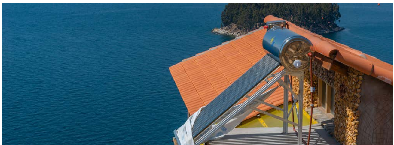
Rooftop solar water heater with hot water storage tank
