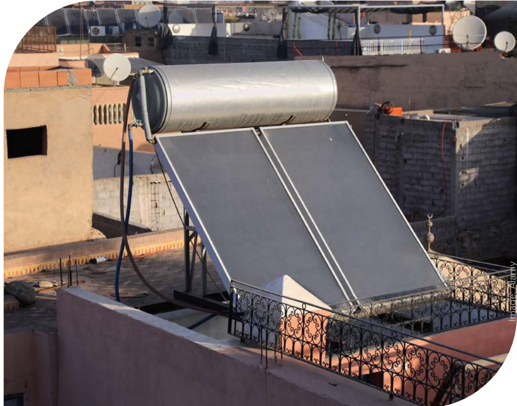
Solar water heater on a rooftop in Marrakech city, Morocco
