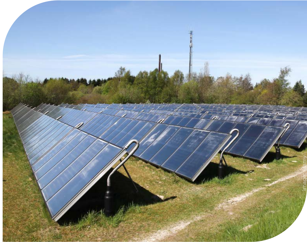
Solar thermal energy panels in Denmark.
