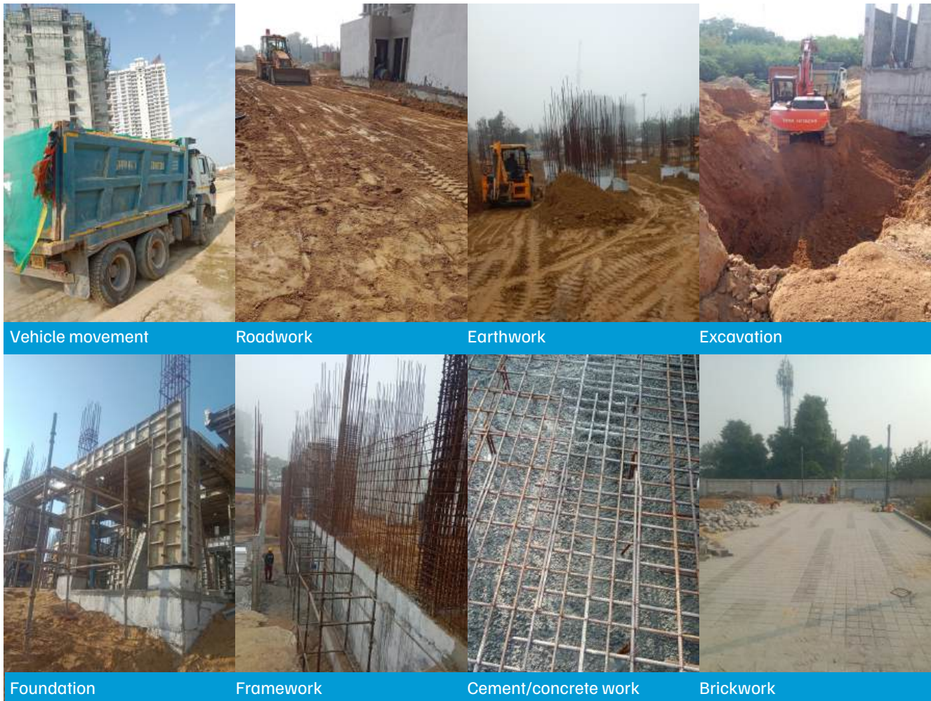
Figure 3. Photos of some on-ground activities taking place at the construction site during the monitoring period
