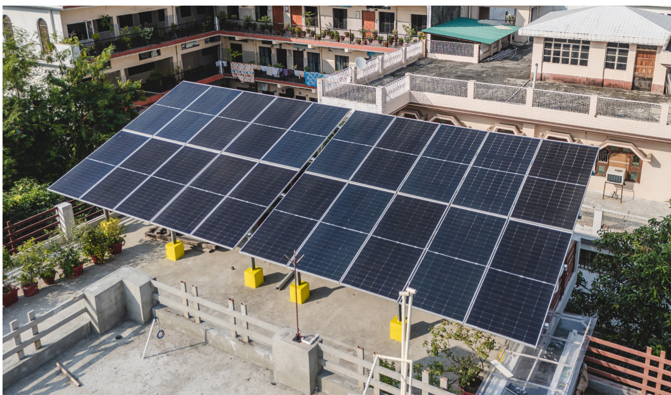
Rooftop solar, Uttarakhand, India.
